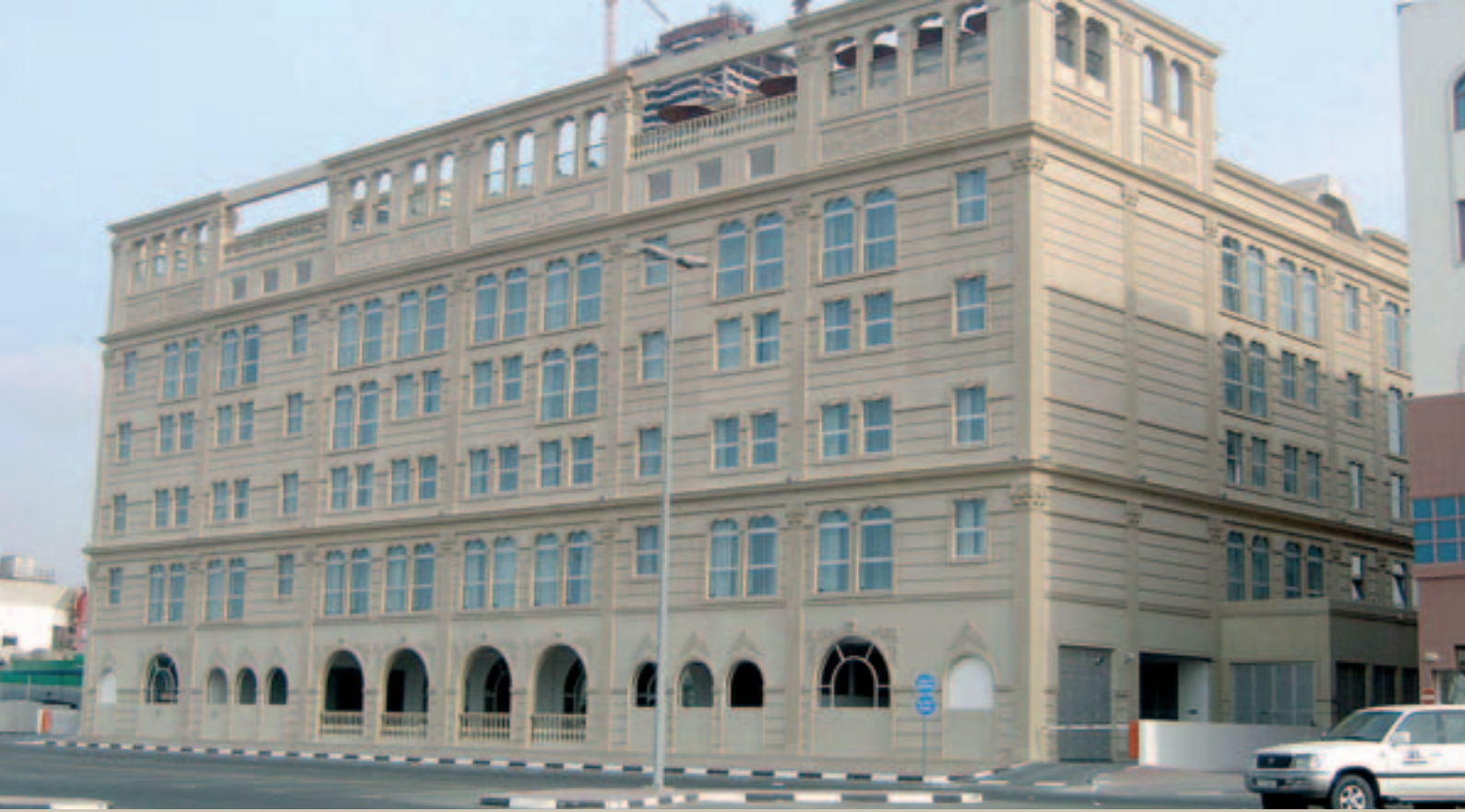
Villa Rotana Executive Apartments is situated on the central Sheik Zayed Road in Dubai. Delivery of columns and beams, hollowcore slabs and insulated wall panels.
