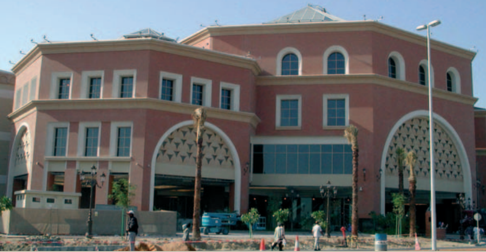
Mall of the Emirates is one of more new shopping malls in Dubai. Some 130,000 sq meters of hollowcore slabs up to 400 mm thick have been delivered.
