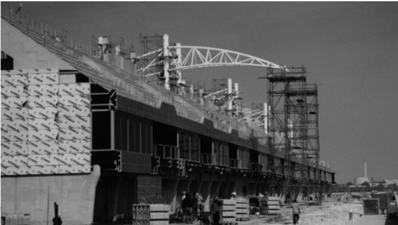
The grand stand at Bahrain's new Formula 1 track has been erected using miles of prestressed Bahrain Precast Concrete panels.
