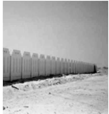
Around each building, a boundary wall is being built. Obviously calling for a precast concrete solution.
