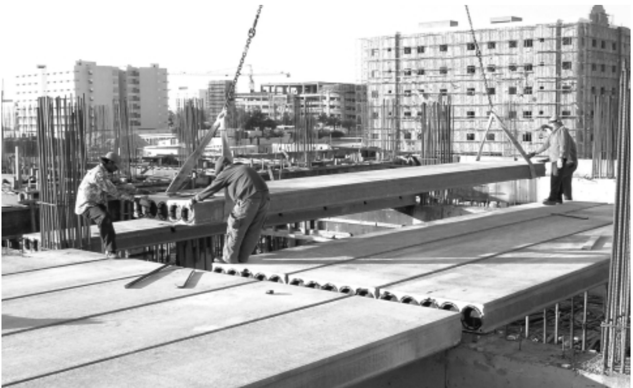
Erection of one of the first hollowcore assignments from the new Qatar plant.
