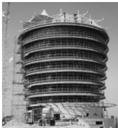
The VIP Tower at Bahrain's Formula 1 track has been erected using Bahrain Precast Concrete hollowcore slabs.
